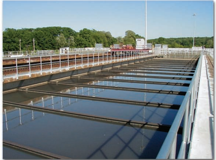
36 ft wide Clarifier - SAV 709 Chain with HMAX Extreme Duty Flights
